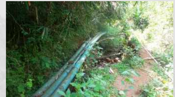
Pipes from irrigation system in Namey village
