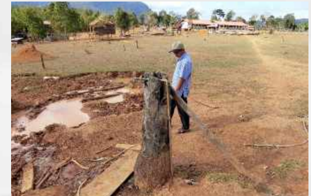
Broken water tap in Fangdeng village
